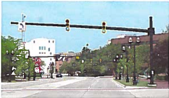
Intersection mast arm
